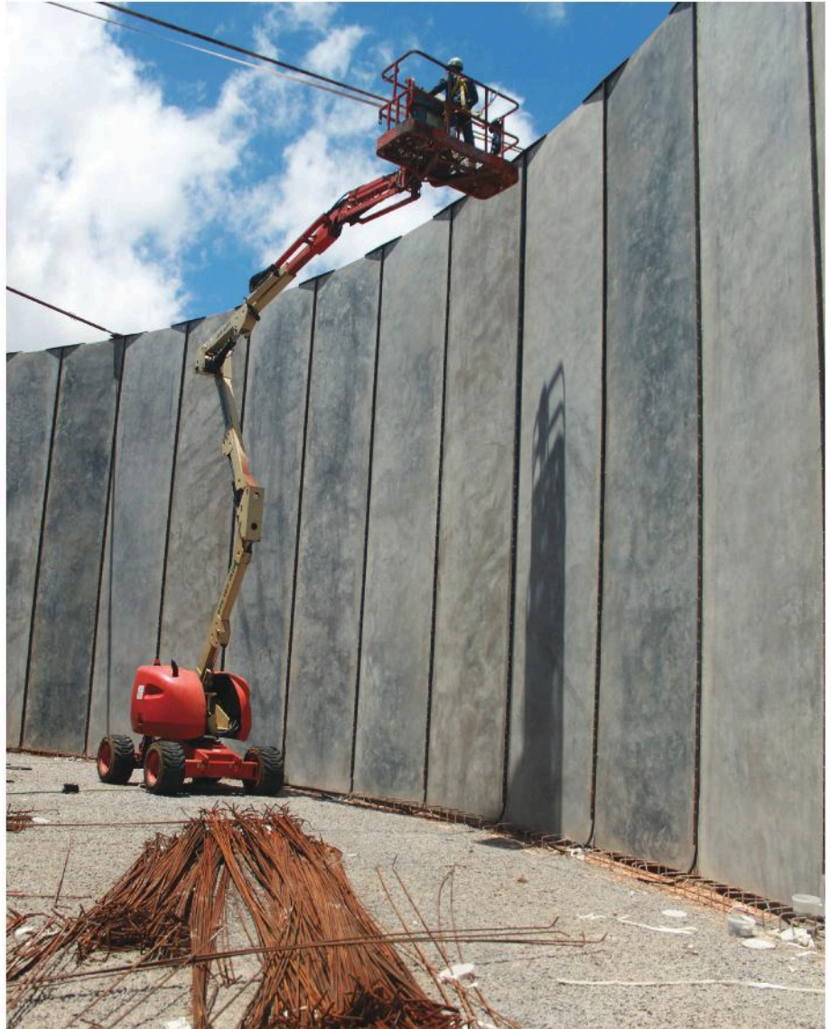
The Corestruc articulating boom lift used to prepare insertion of grouting between the panels.
